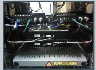
One of NIW's installed base stations
